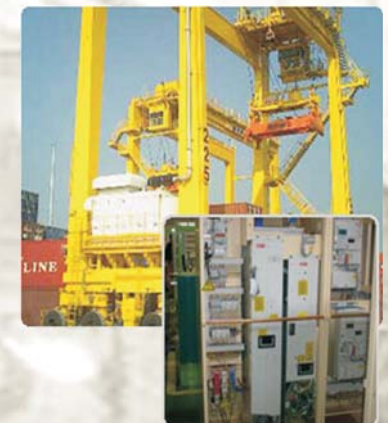
CRANE SYSTEM PANEL
